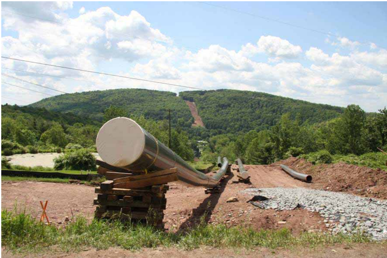
The Millennium Pipeline will allow for increased amounts of natural gas to be transported in New York State. (Photo by David B. Soete)
