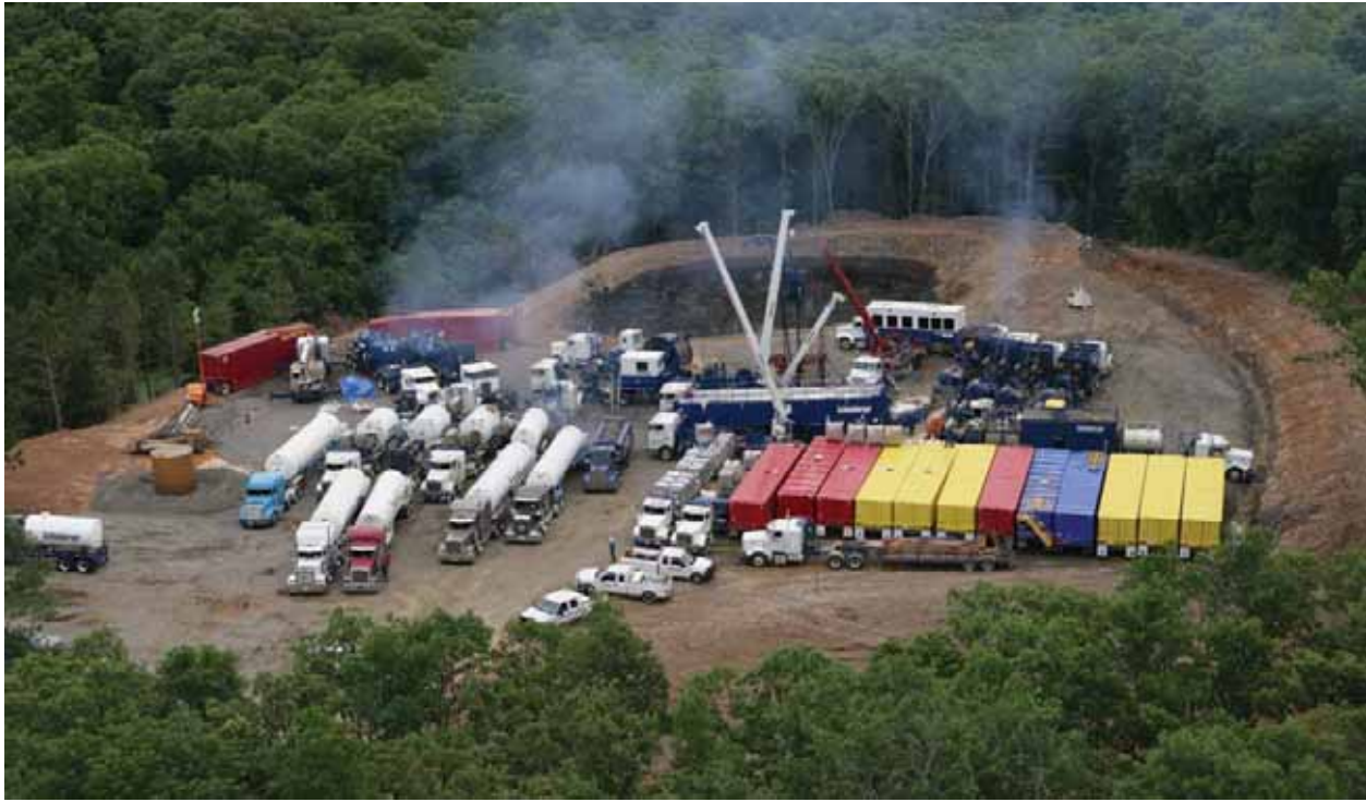
The numerous truck-mounted pumps and temporary storage tanks needed to fracture-treat the Marcellus Shale will require larger well locations. The fracturing equipment and materials on location in this photograph represent over 100 round trips to location by large tractor trailer trucks. (Photo source—Unknown)
